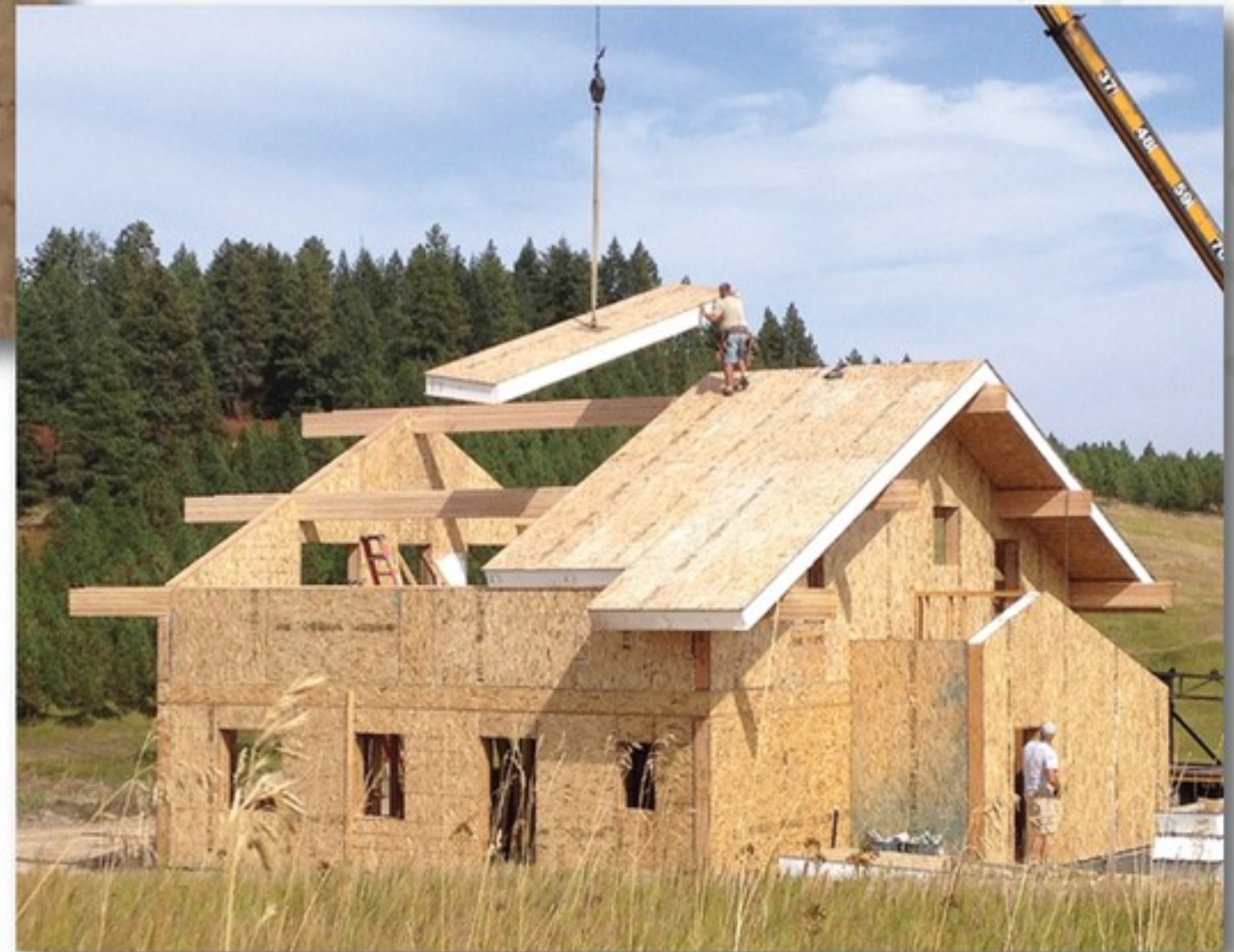
▲ Compared to traditional stick-frame construction, assembly of the panels on-site saves enough time and labor to make SIP a competitive cost-effective solution.
